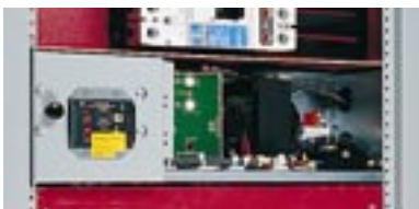
Branch circuit breaker ground fault protection can be provided integral to the device or with separate relay and test panel mounted in compartments similar to the circuit breakers for convenience and space savings.
